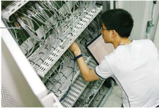
FIGURE 8.7 A wiring closet enables an IT technician to make adjustments to several connections from one location regardless of where the devices are located.
